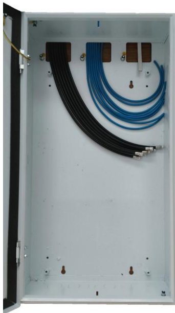
Enclosure with Coax and Data cables installed
