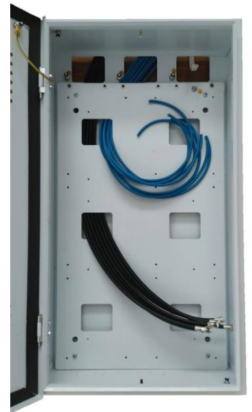
Enclosure with Gear Tray reinstalled and cables directed to their locations ready for frame and module installation.
